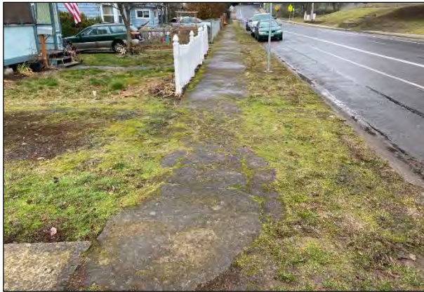
Figure 3-6. Example of Deteriorating Conditions on a Local Sidewalk
