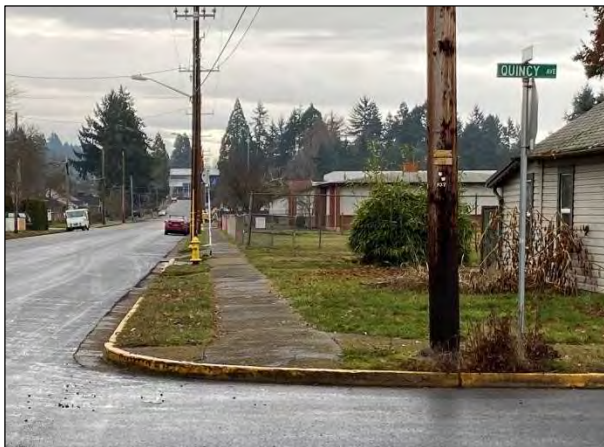
Figure 3-8. Missing Curb Ramps along Quincy Avenue
