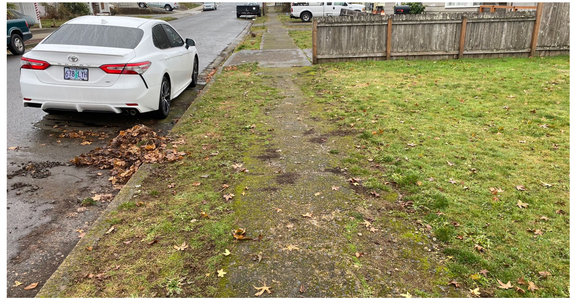
Example of Excessive Weed Growth on a Local Sidewalk
