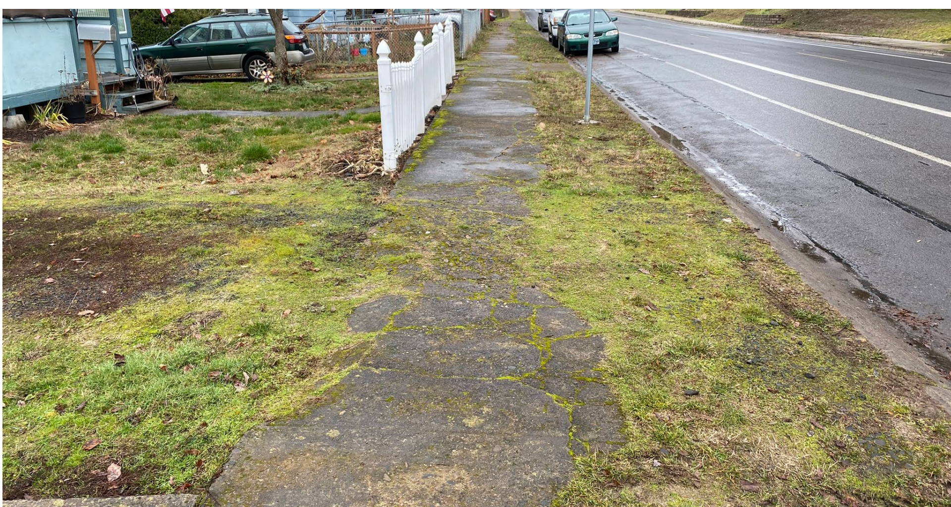
Example of Deteriorating Conditions on a Local Sidewalk
